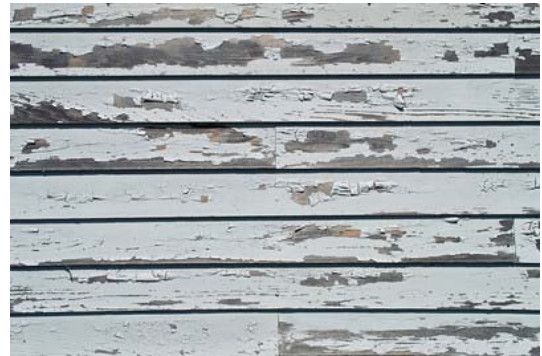
Most original wood siding can be brought back to good condition once it has been properly treated.
